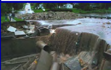
D. Water Control Facilities
